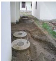
SEPTIC TANK (ON-SITE SANITATION)
